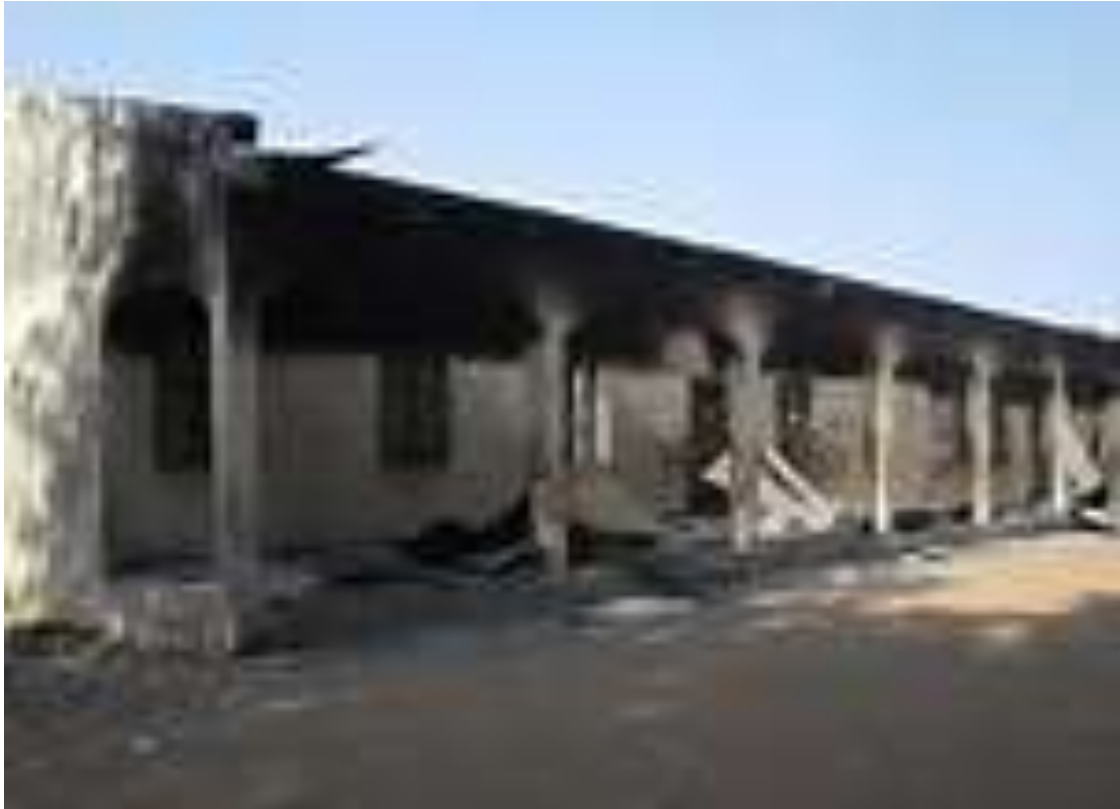
Figure 2 One of the destroyed parts of Kulogumna Primary School
