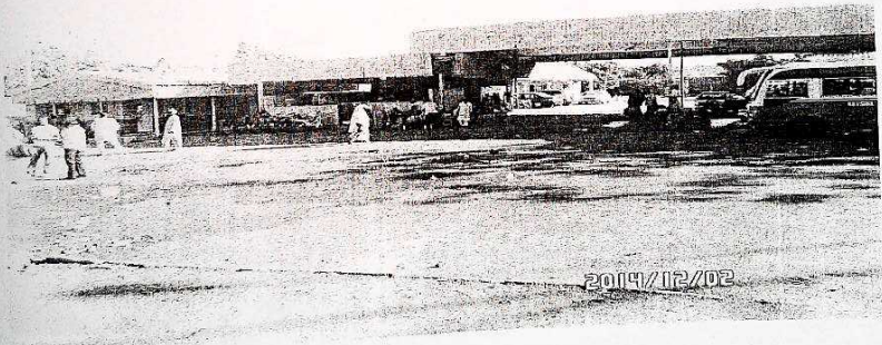
Plate: 3.2 Lack of proper drainage in the terminal.
