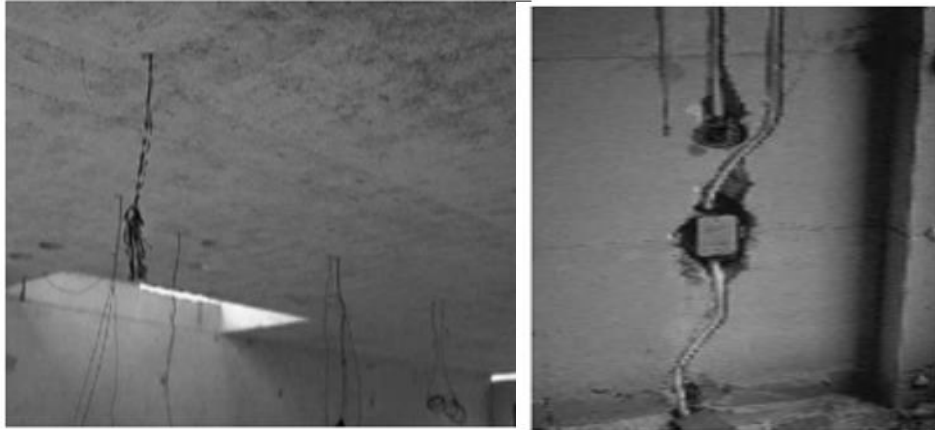
Plate IX: Cables and Pipes Housed in Weight-Bearing Floors (left) and Walls (right). Source: World Building Congress, 2016
