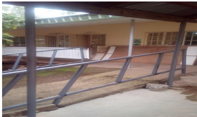
Plate XXXV: Department of Nursing Sciences, Showing the Method of Construction. Source: Author's fieldwork, 2016
