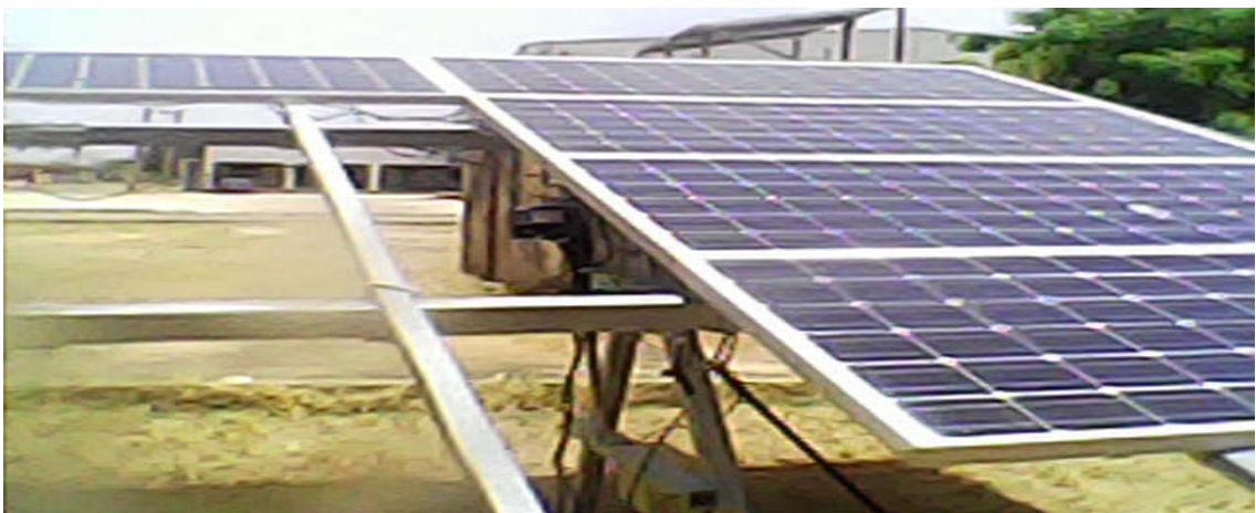
Figure 3.14 Developed System Connected with PV System Panel
