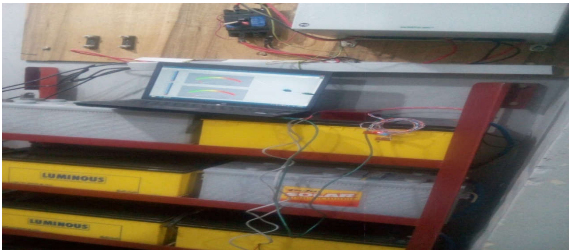
Figure 3.13 Developed Monitoring System Connected with PV System Power Bank
