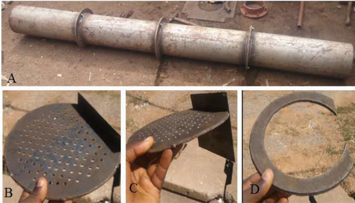
Plate 4.5: Image of Stripping Column (C-100) and its Internals During Fabrication
