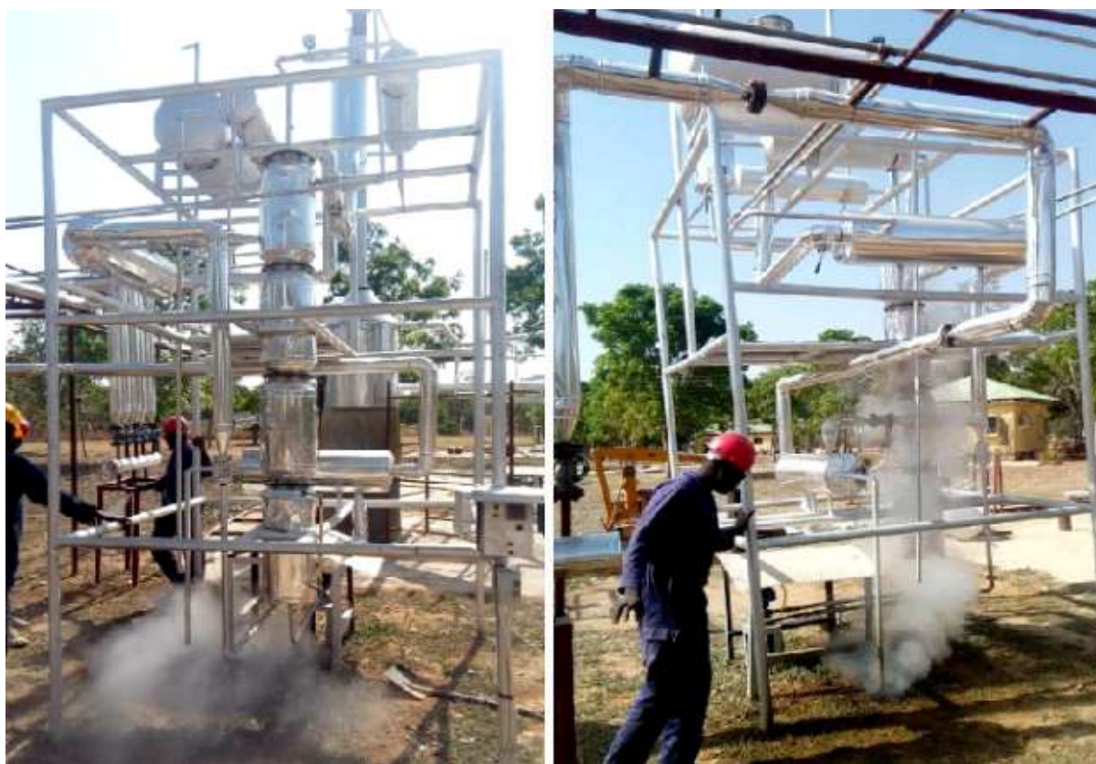
Plate 4.10: SWS Unit During Test Running.
